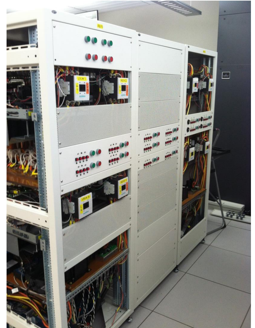
CURRENT's HTB Area cabinets use inverters to represent sources, lines, loads, and storage
