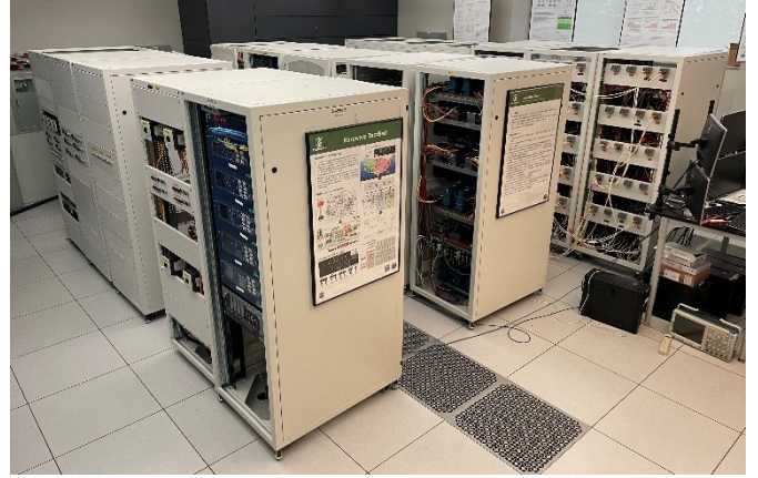
Fig. 7. Power converter-based hardware test bed (HTB).
