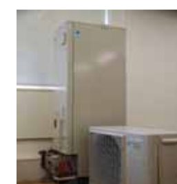
HP Water Heater
