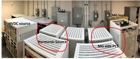
Fig. 8. PCS APF testing hardware setup.
