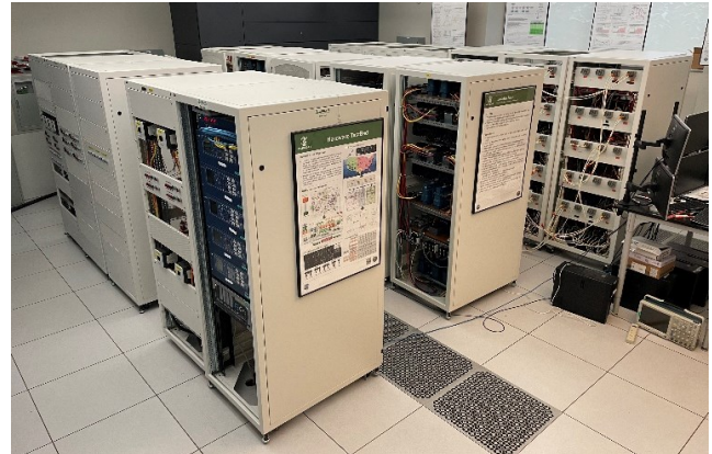
Fig. 7. Power converter-based hardware test bed (HTB).
