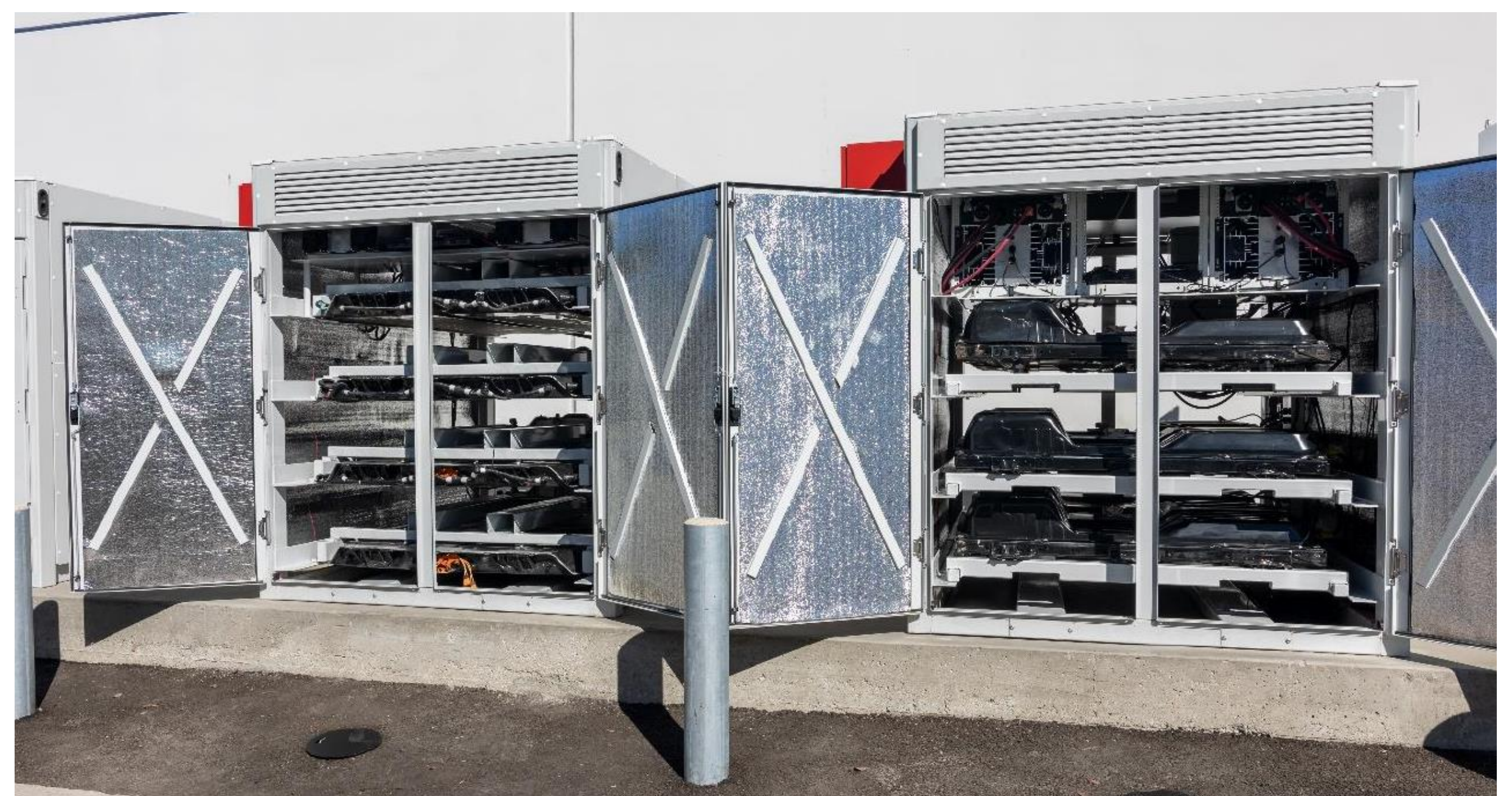
Fig. 3. Battery Energy Storage System Left Housing 4 Tesla Battery Packs, Right Housing 4 Nissan Leaf Battery Packs
