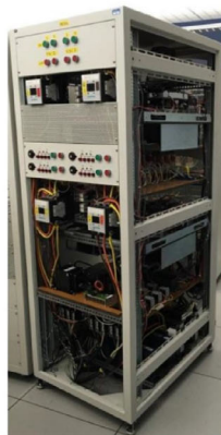
(c) CURENT Hardware Testbed cabinet with inverters and filters
