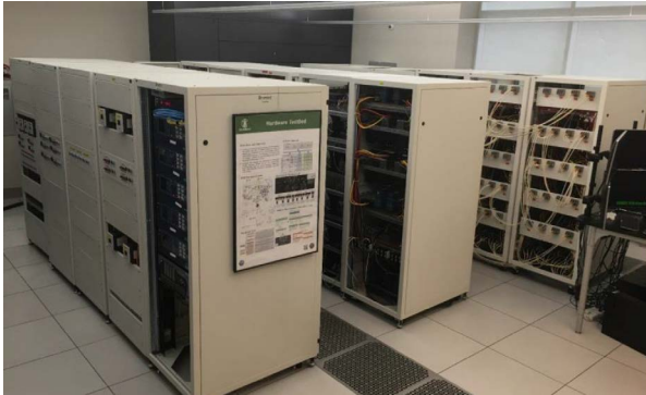
(a) Converter-based HTB cabinets
