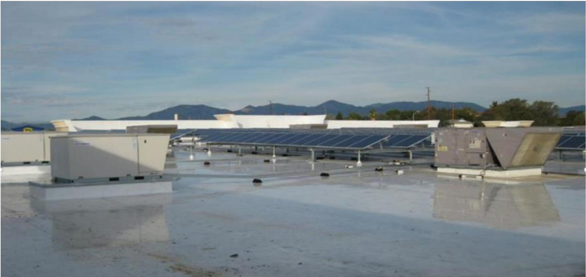
Utility, Large Big Box Retail, Solar & Storage Project
