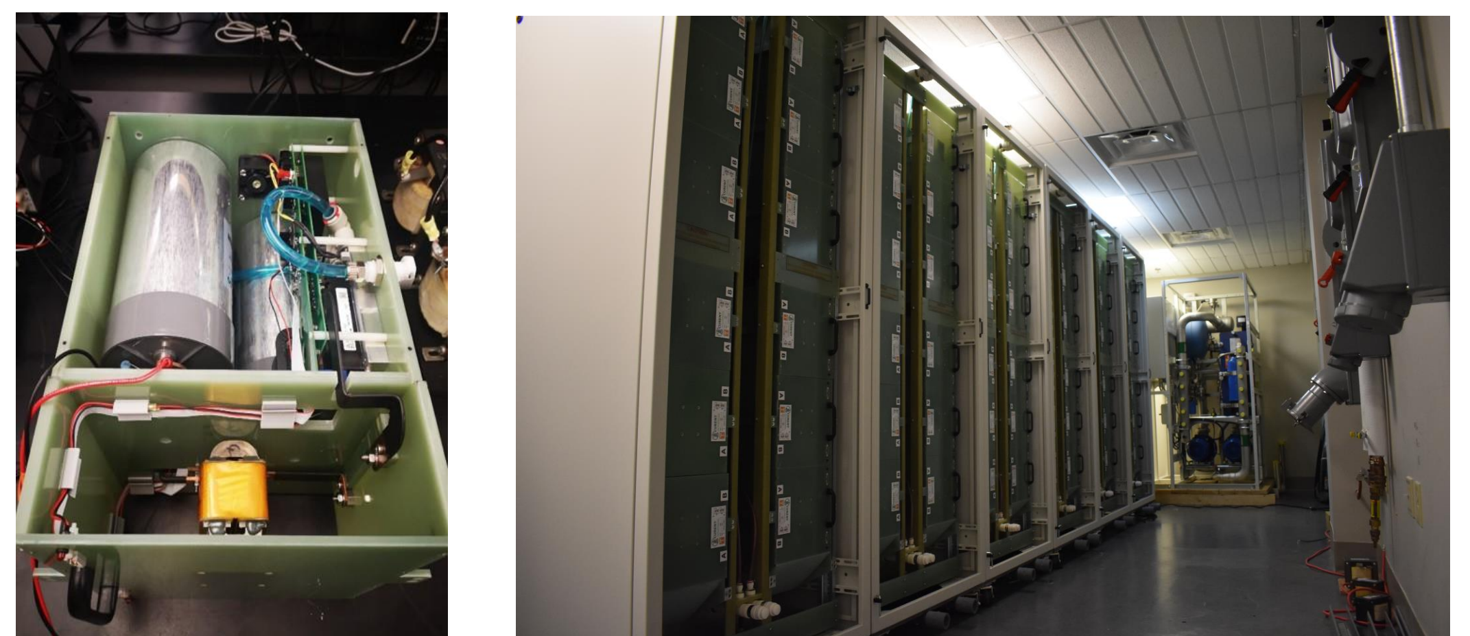
Fig.4 Full scale module and power cabinets.
